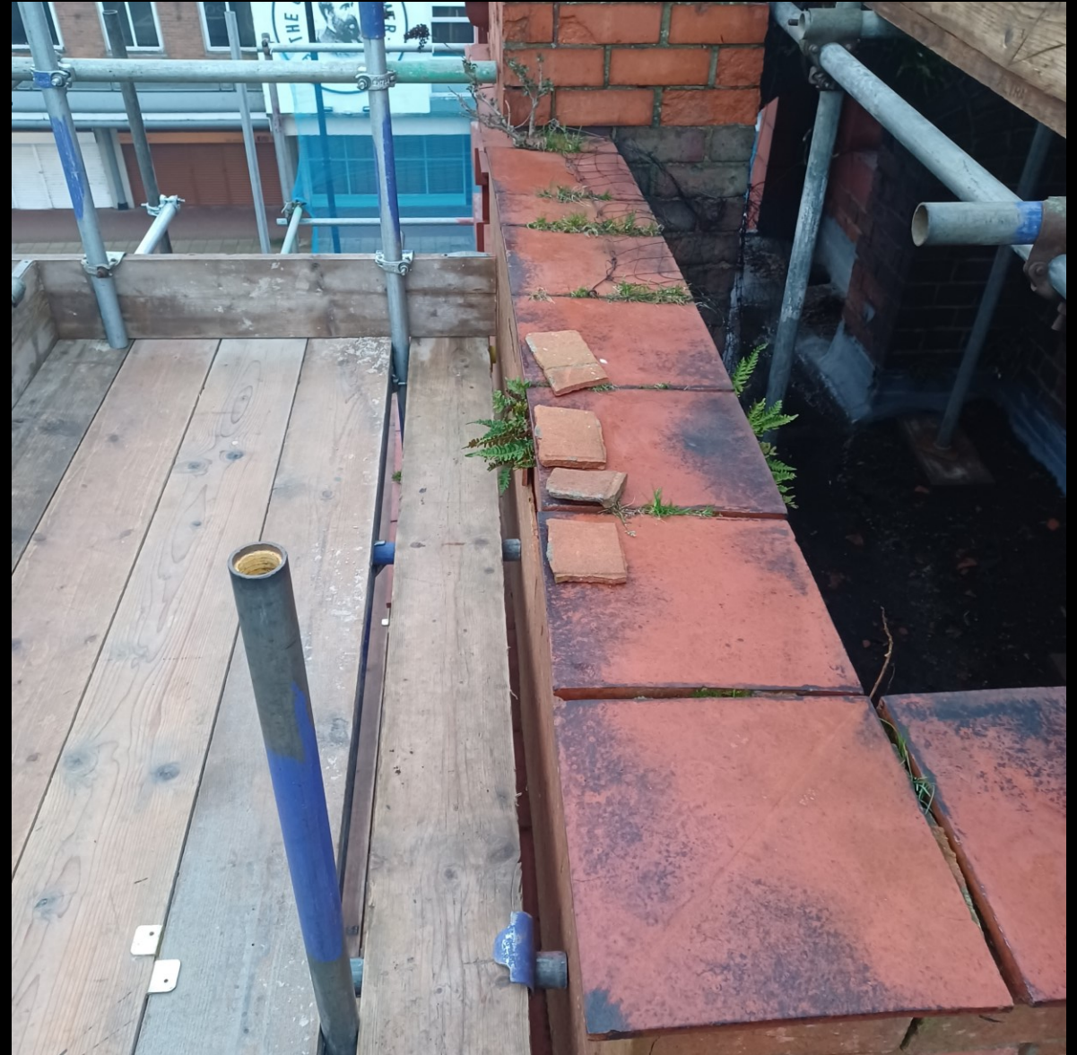
Side elevation, capping to parapet wall, showing failed render
