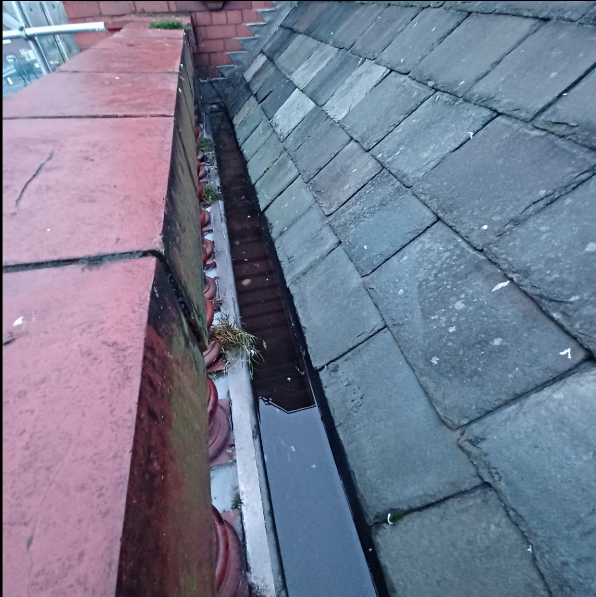
Blocked gutter behind balustrade / parapet wall
