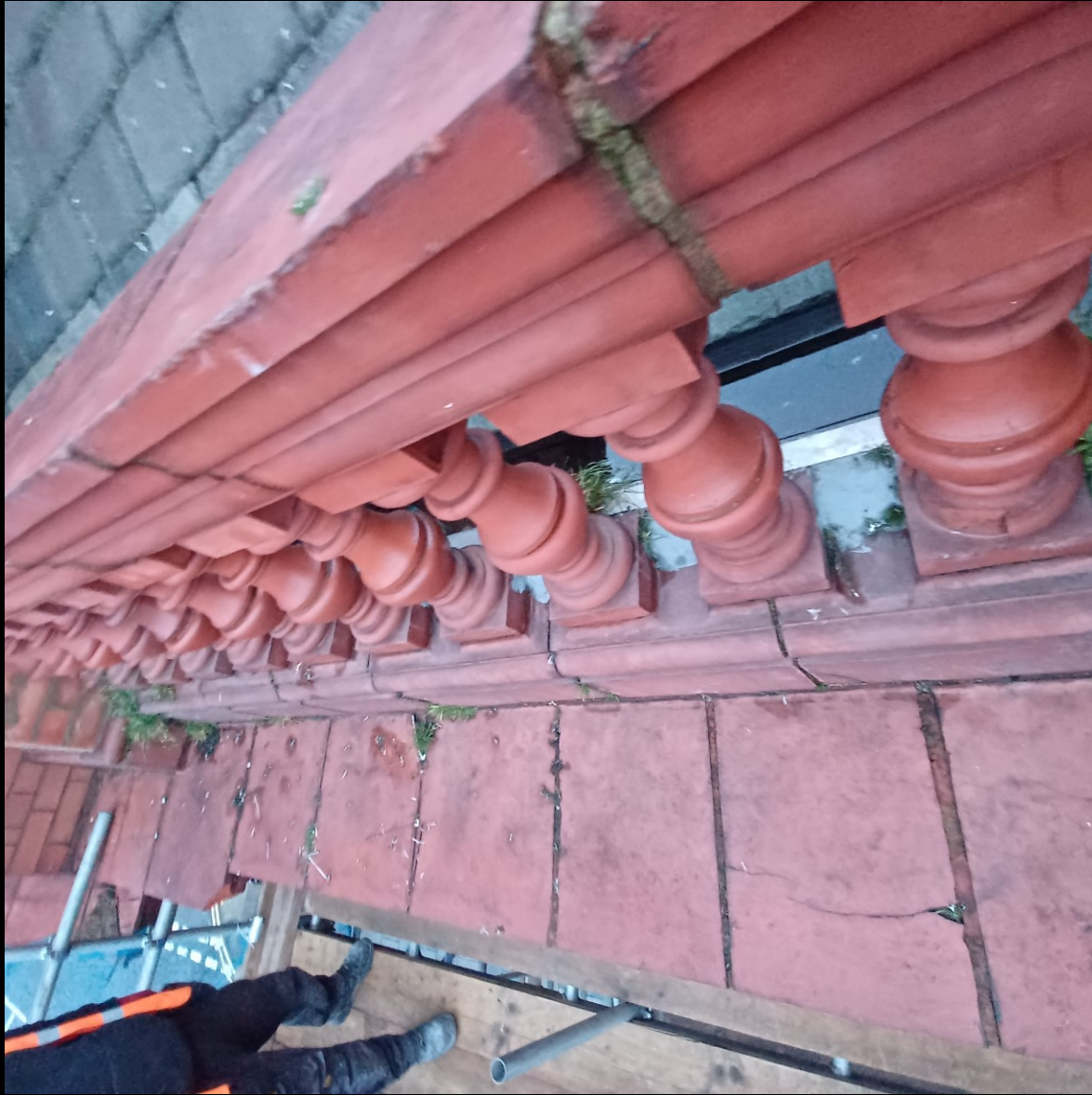
Balustrade / parapet wall with vegetation to joints and blocked gutter
