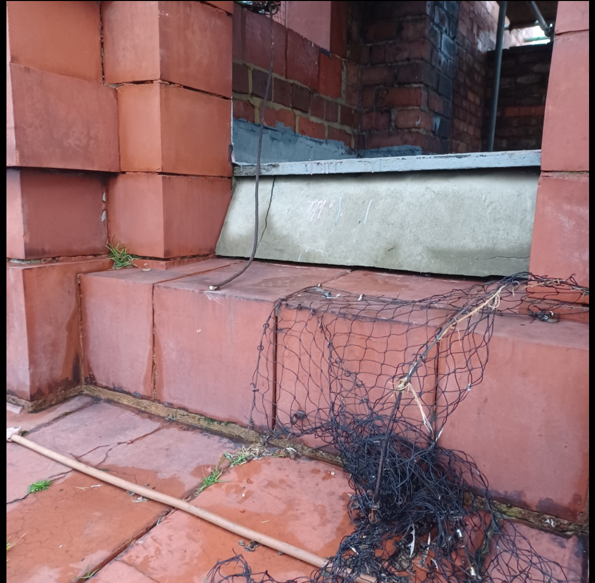
Joints with vegetation and ineffective water diversion inside small arch. Later addition. Also note failed netting
