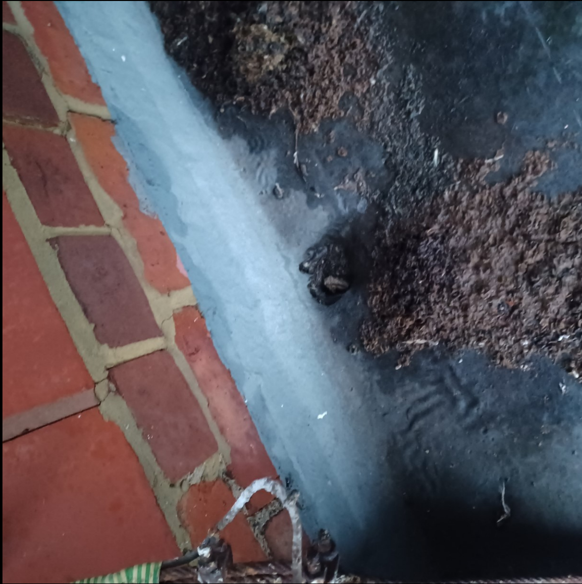
Debris blocking outlet to rainwater good, causing water ingress into building
