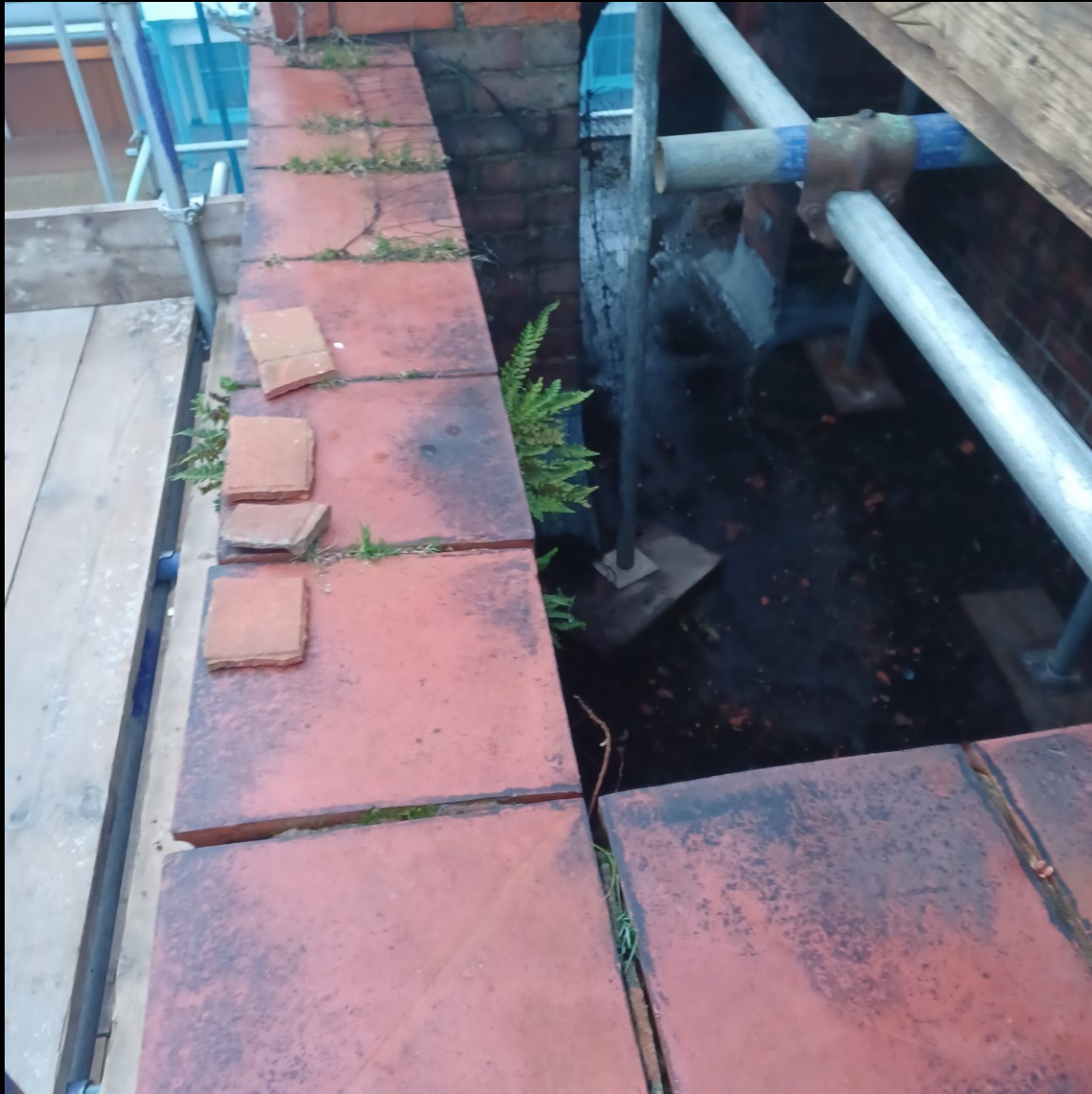
Front Elevation, Parapet wall, with loose capping stones and vegetation in joints
