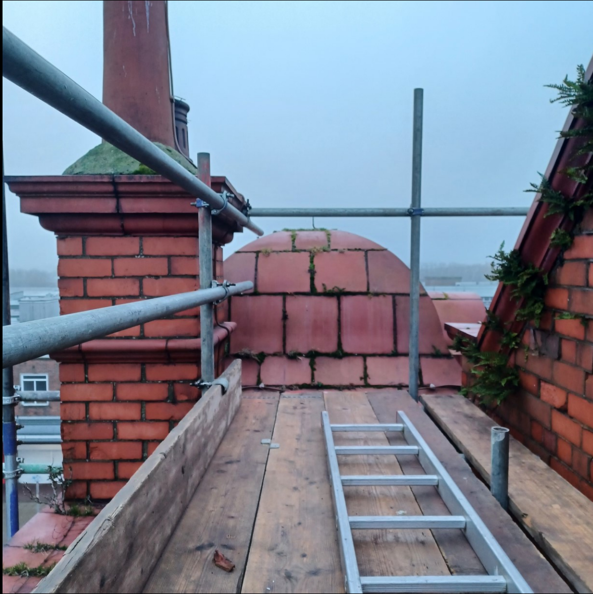
View from rear of small arch, showing vegetation growth in all the failed joints
