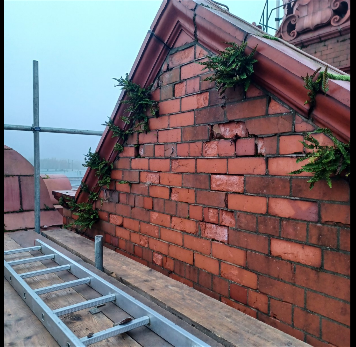
Side elevation with patched failed render and vegetation
