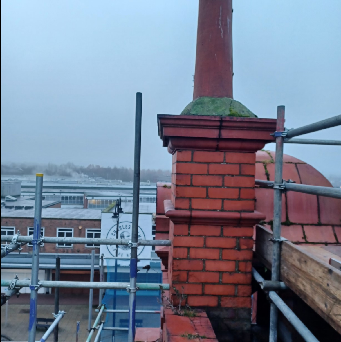
Chimney with failed haunching
