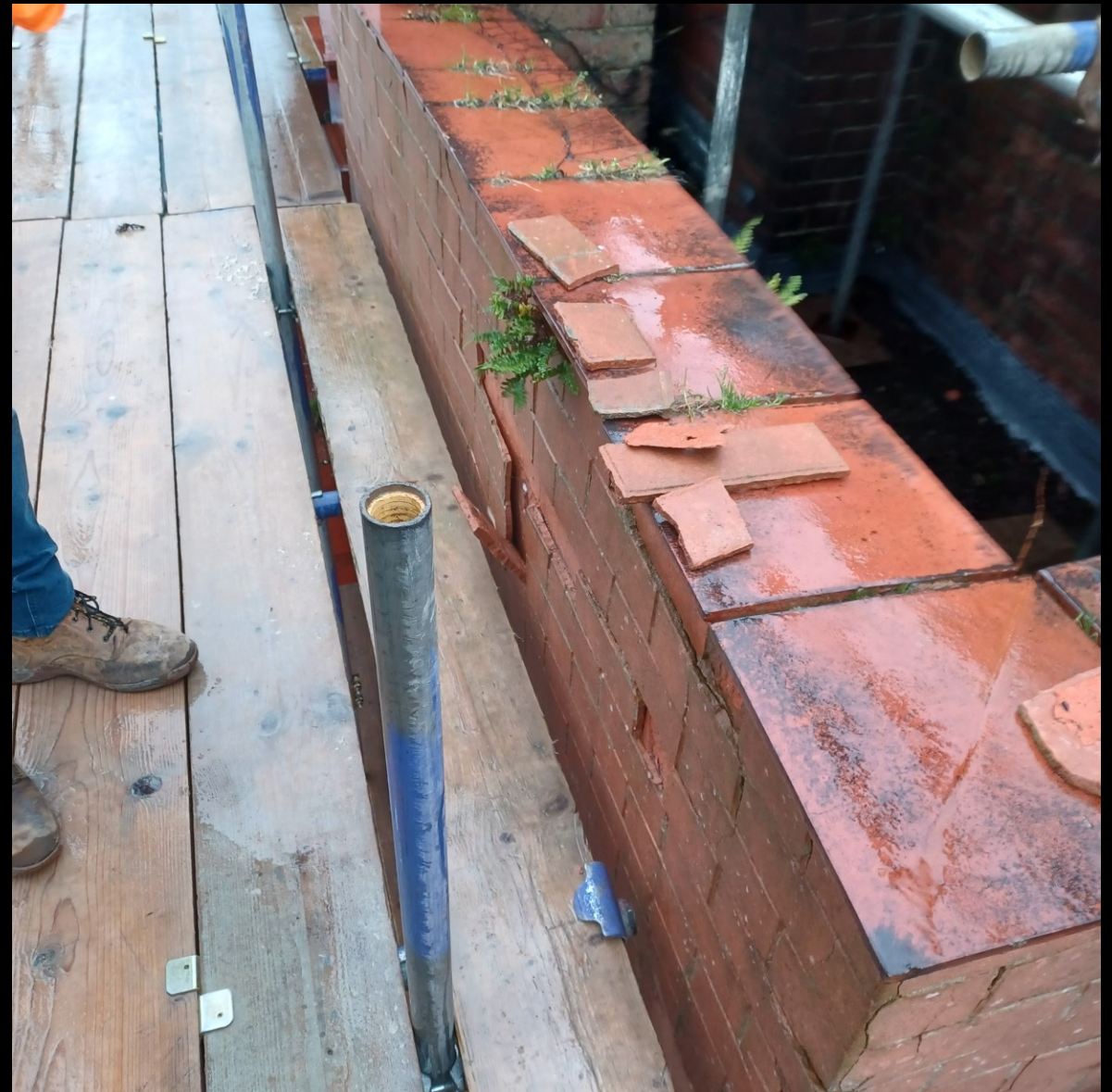
Small Parapet wall showing loose capping and failed render
