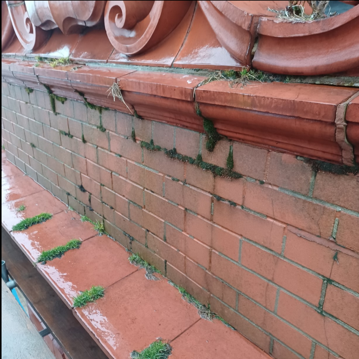
Front Elevation – vegetation growth and gaps to joints
