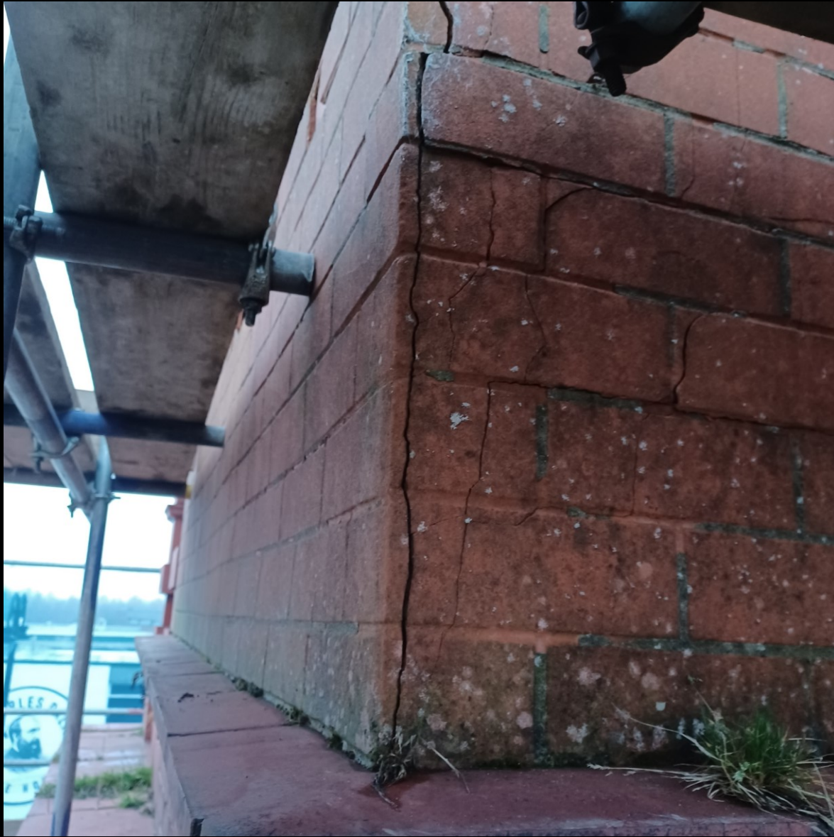
Failed Render to small parapet wall behind small arch. Also note vegetation to joints.
