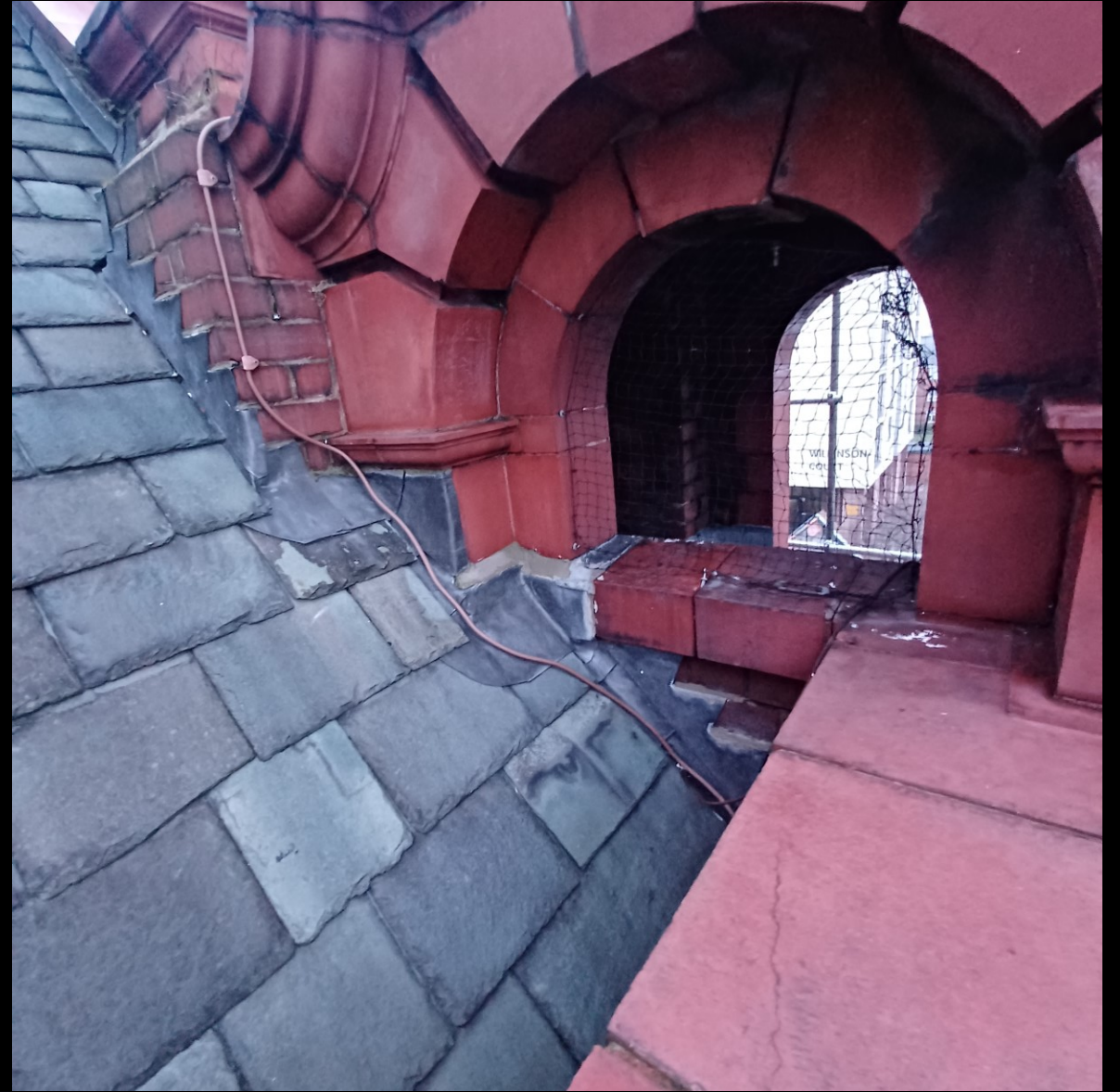
Small decorative arch with vegetation to joints and failed netting
