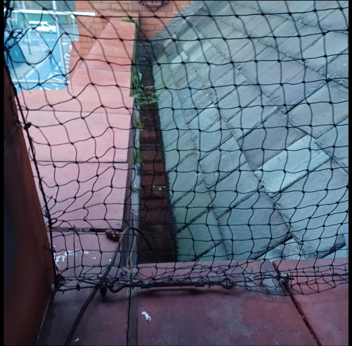
Blocked gutter causing water ingress into building
