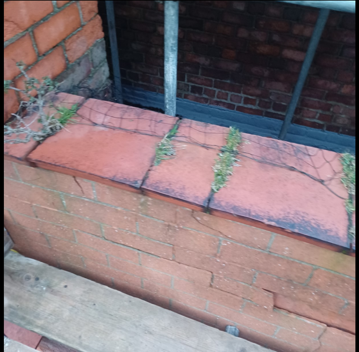
Parapet wall with failed render, loose capping stones and vegetation
