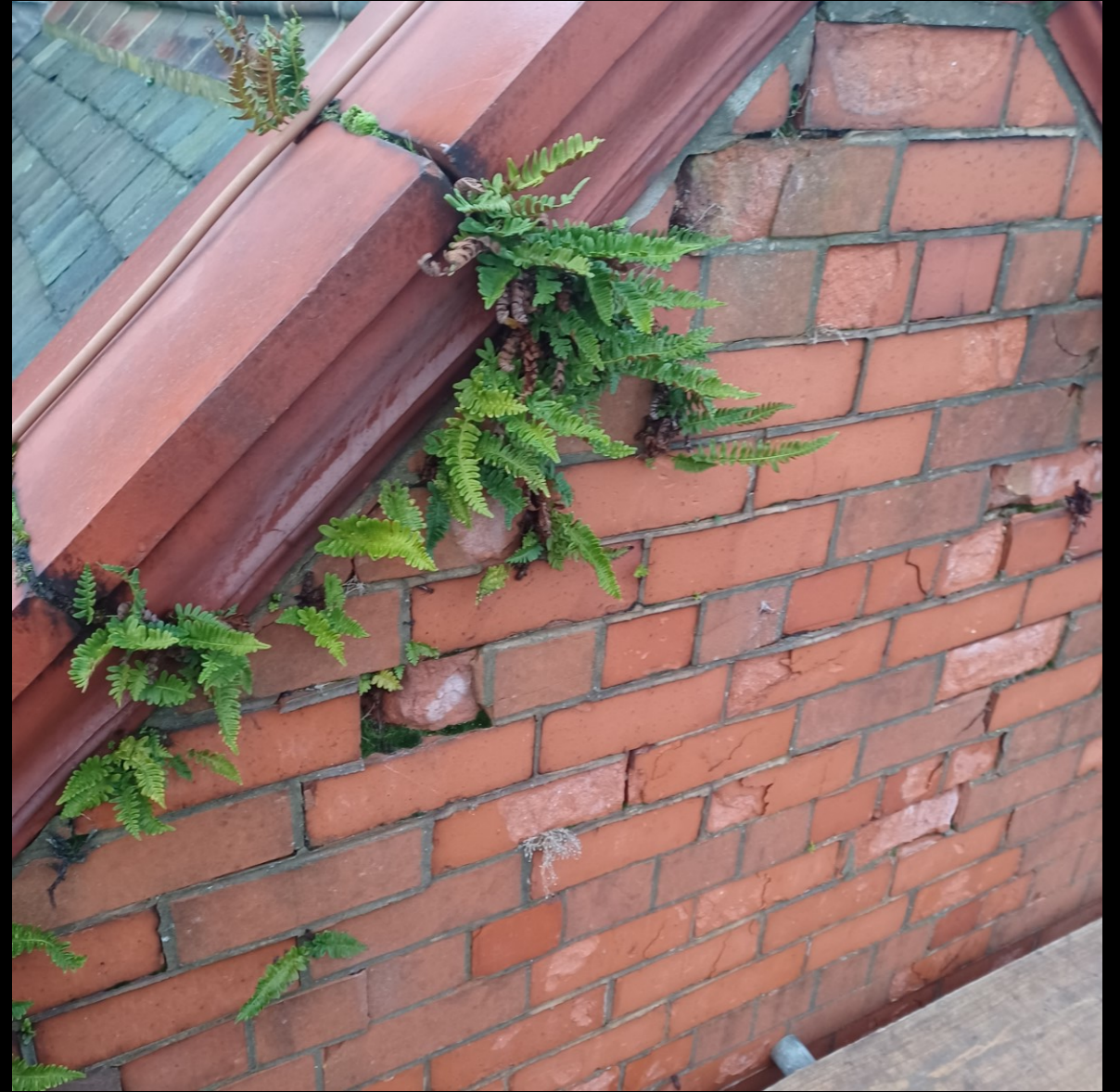
Gable end showing vegetation to failed render
