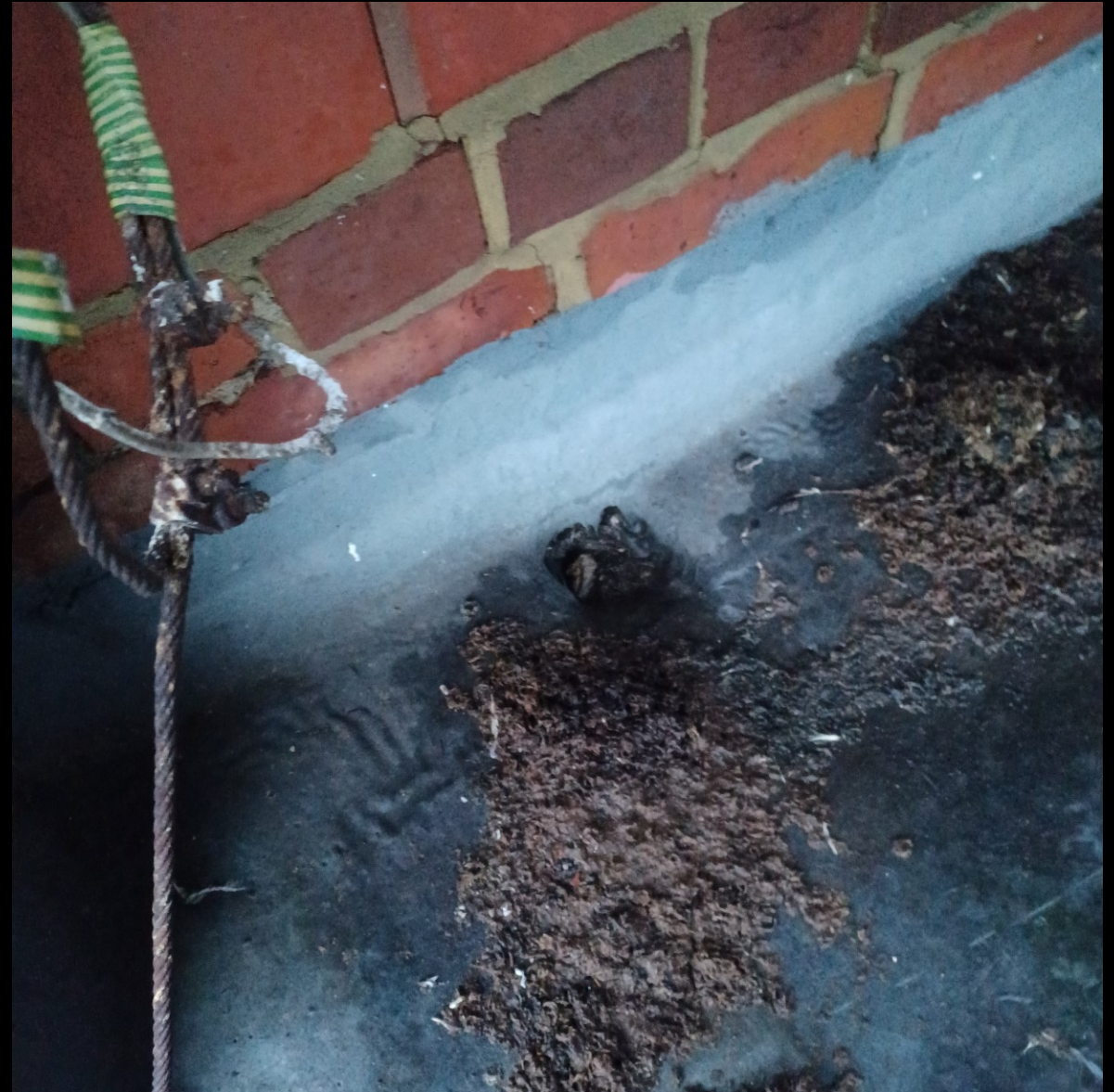
Side Elevation, behind small arch / parapet wall. Debris blocking out to rainwater goods
