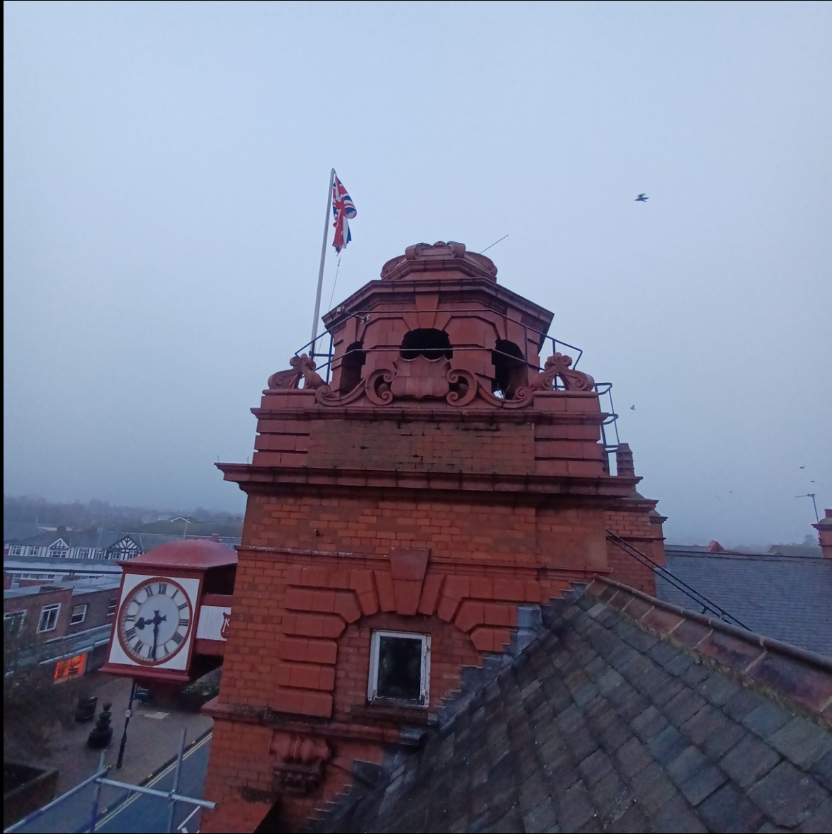
Main Tower with patch render repairs, failed / damaged brick work and vegetation growth to joints
