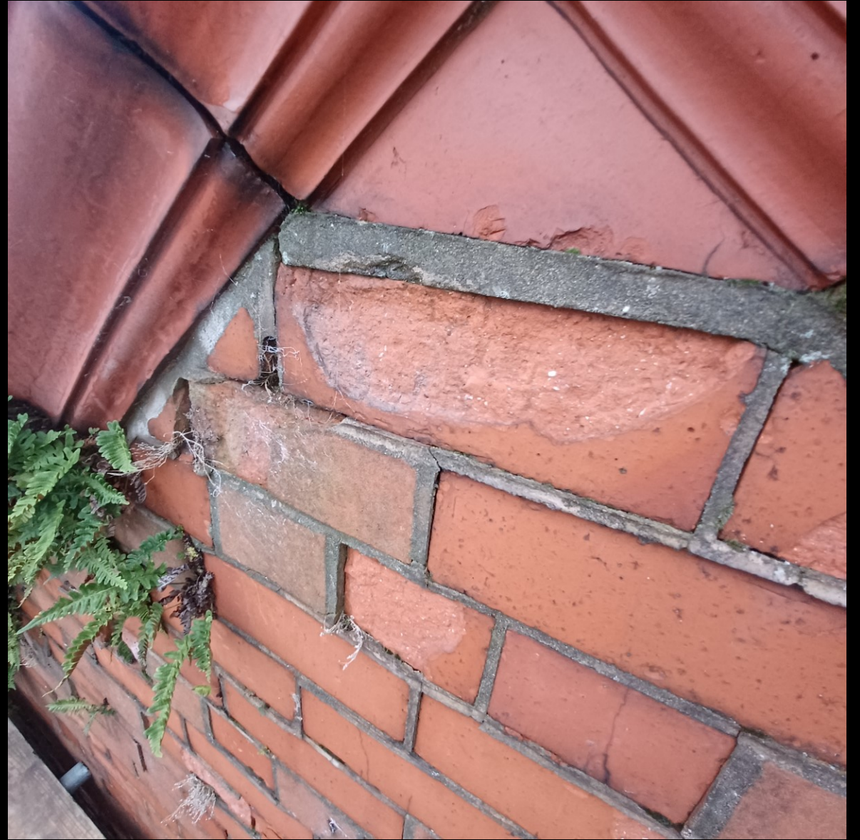
Gable end with vegetation growth and failed render / damaged brick work
